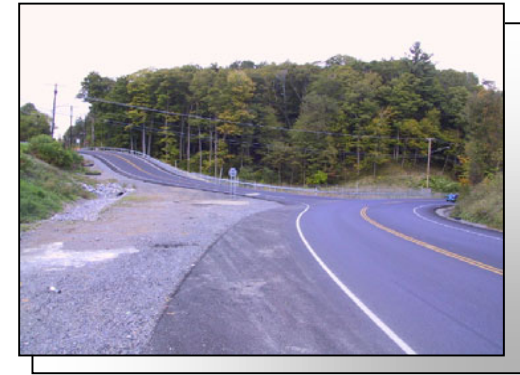
The profile was raised, the median was removed, and the horizontal and vertical alignments of the spur were improved.
